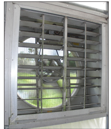
Figure 8. Although fans are important for temperature control, they can spread disease-causing organisms by blowing contaminated water bubbles throughout a facility.
