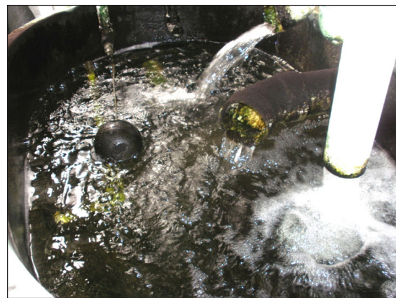
Figure 5. Sump from RAS. Depending upon design, sumps can build up significant amounts of debris, which can harbor disease-causing organisms. Sumps require periodic cleaning.
